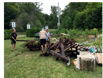
It took heavy equipment and many pairs of hands, plus lots of time, money and effort, to dispose of the derelict docks.
